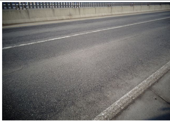
S11 망상균열 (원주방향)
